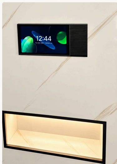
Smart control panel above a lit niche.
